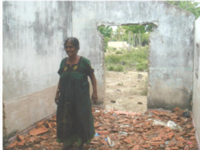
A Resident of Pungudutivu, Jaffna shows us a damaged house
